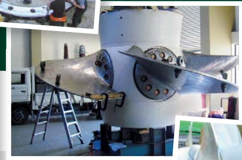
Overhaul of large Kaplan Turbines. Refurbishment and manufacture of small Kaplan Turbines
